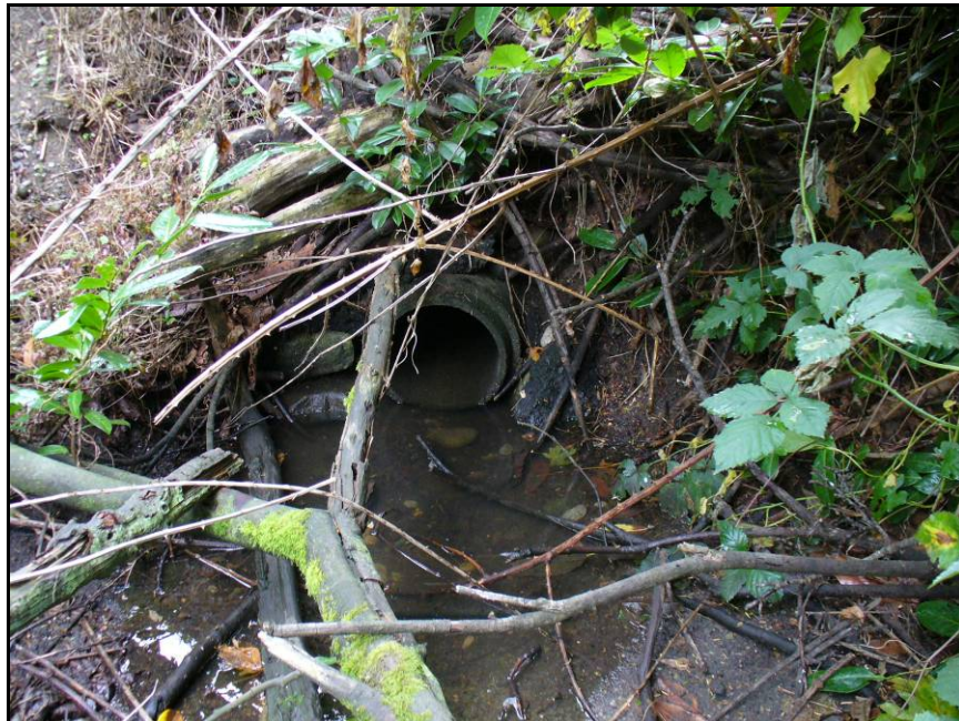
Photo 1, 12-inch-diameter concrete pipe stormwater outlet culvert below NW 180 th Street (Oct. 2, 2008). Puddled water at the outfall does not extend downslope.
